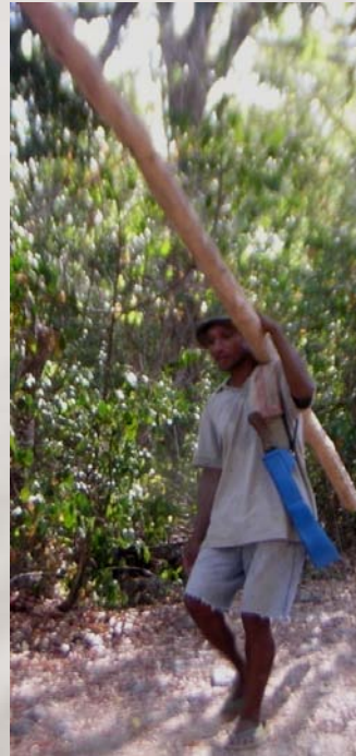
Selected timber from nearby bush was manually cut and carried to the site
