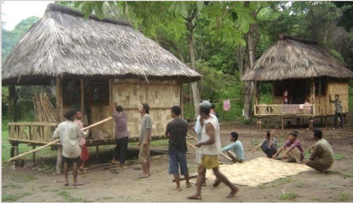
The two lodges almost completed with roofs made from coconut leaves fastened with palm fibre
